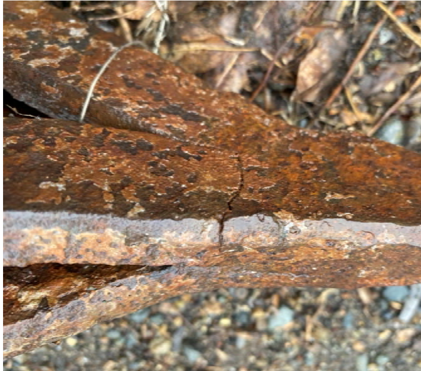
Figure 12: Cracks in Lateral Bracing Rods
