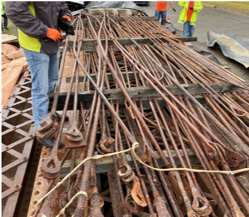
Figure 14: Lateral Bracing Rod Deformations
