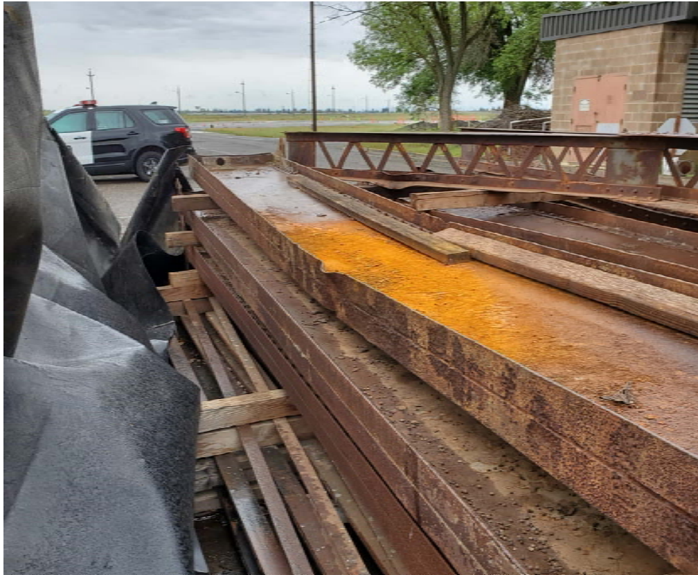
Figure 7: Rusted and Deformed Floor Beam Member
