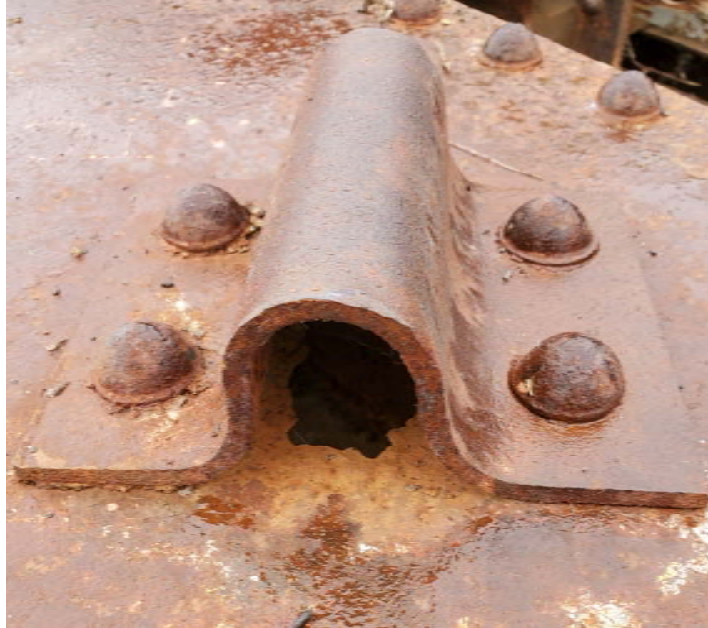
Figure 8: Hole in Top Truss Chord Plate
