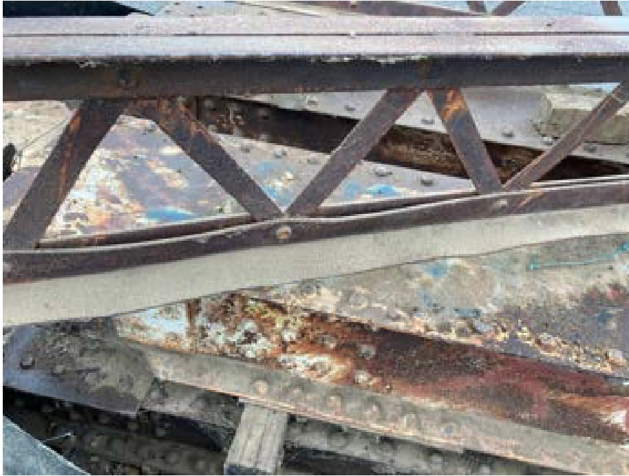
Figure 11: Portal Beam Flange Deformations
