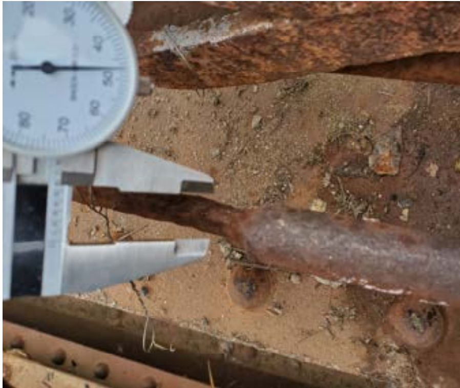
Figure 15: Major Rusting of Lateral Bracing Rods
