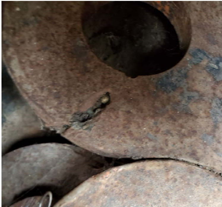
Figure 10: Damage in Straps and Bottom Chords
