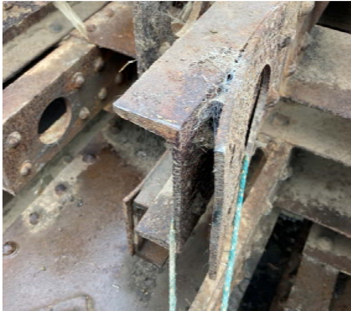
Figure 9: Diagonal Chord Web and Additional Plate Separation
