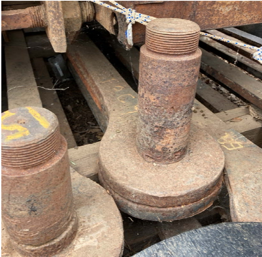
Figure 17: Cut Pin Connections Stuck in Members
