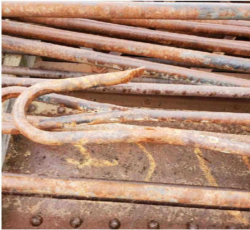
Figure 13: Broken Lateral Bracing Rod Connections
